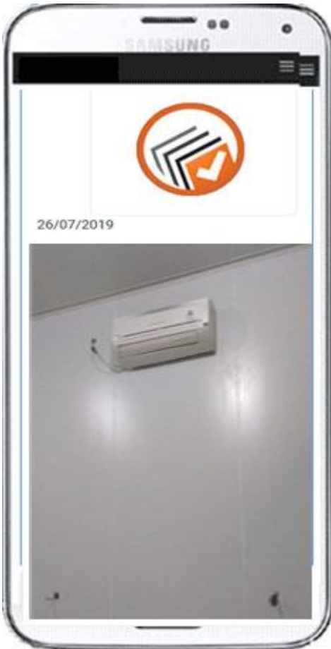
Take and upload photos of issues identified during monthly inspections
